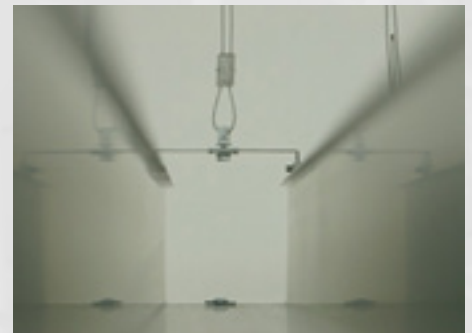
Image displaying adapter and wire suspension in-situ, offering a mechanical fix to the services which are secure and level.
