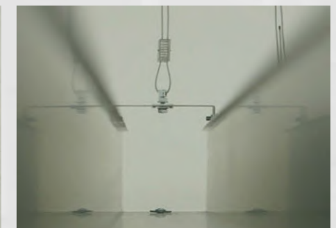
Image displaying adapter and wire suspension in-situ, offering a mechanical fix to the services which are secure and level.
